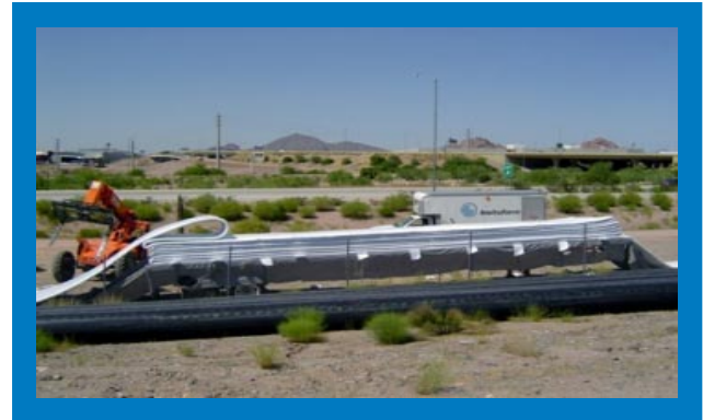
To repair large diameter concrete pipe, new liners were created by impregnating miles of Insituform® felt with Vipel® resin. (Image is used courtesy of Insituform Technologies, Inc.)
